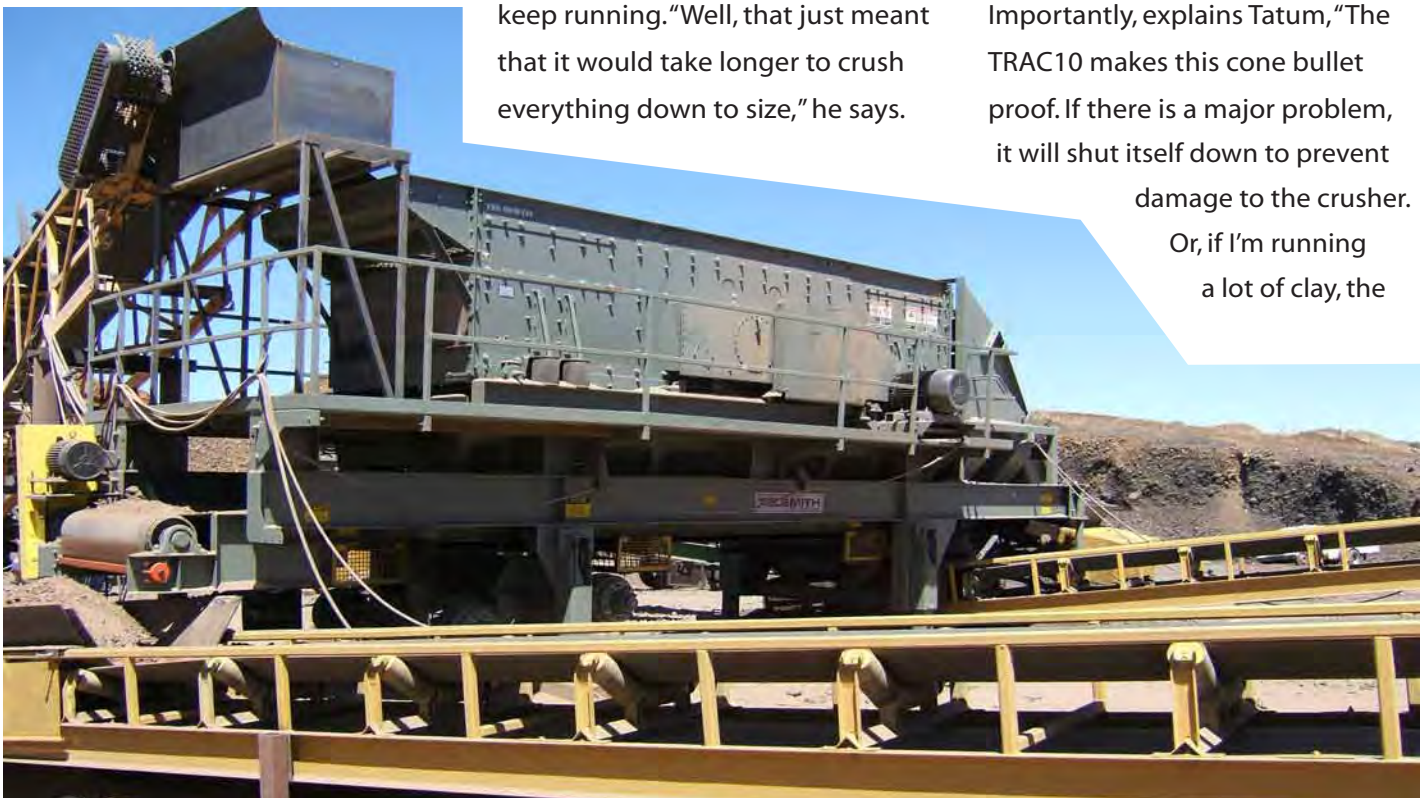
A Telsmith 6' X 20' triple deck horizontal screening plant sizes stone for stockpiling.
